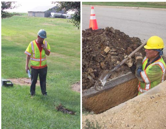
Workers at the other end of the site guide the cable progress. At right, depth of a water main is checked prior to cable being bored.
