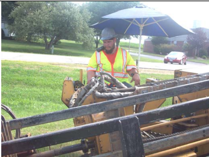
A worker from PirTano Construction Company runs the fiber optic cable boring equipment.
